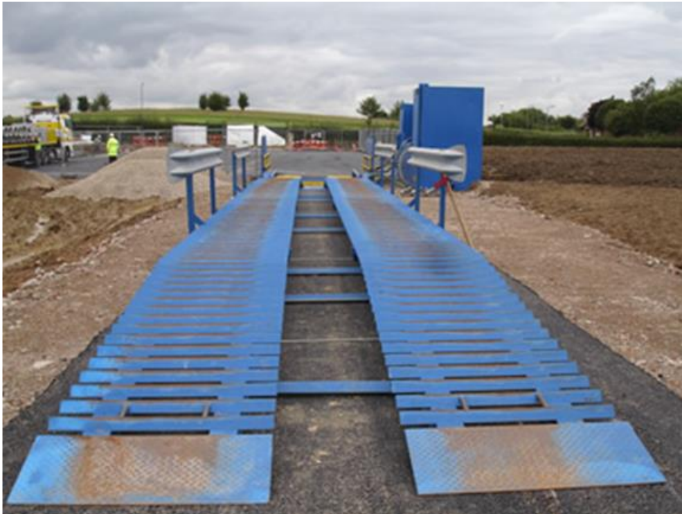
Plate 11: Example of a dry ramp wheel wash facility
